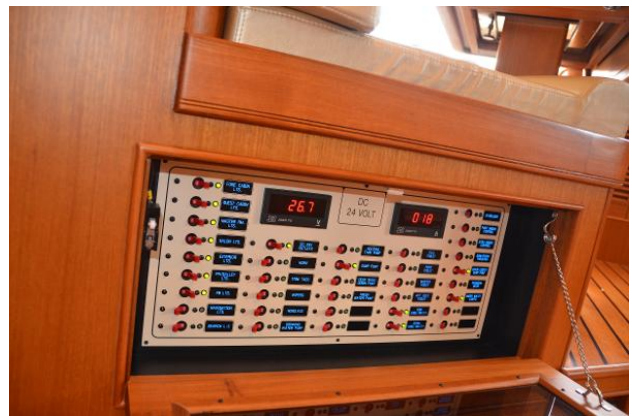
24V Electrical Panel
