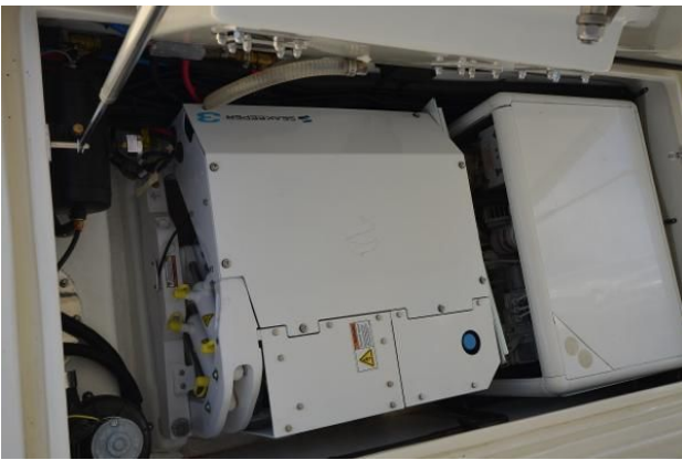
Sea Keeper and Generator
