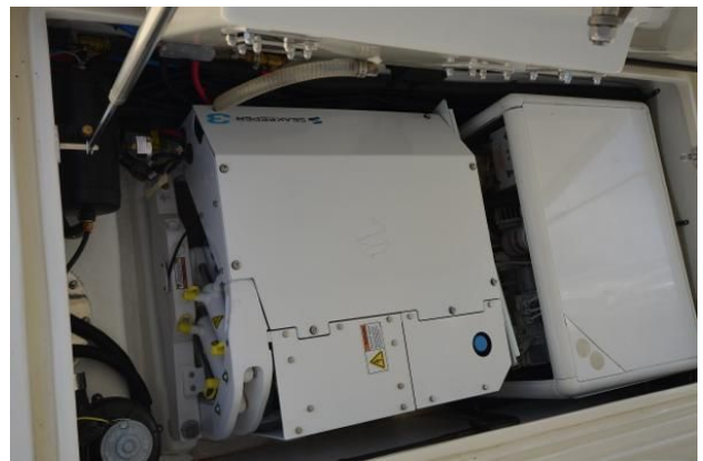
Sea Keeper and Generator
