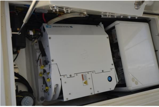
Sea Keeper and Generator
