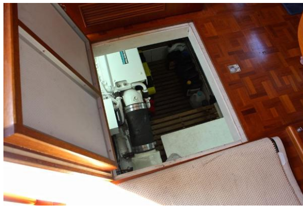
Salon engine room access
