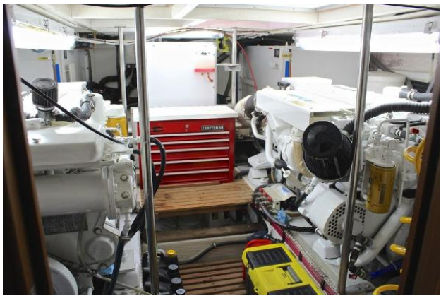
Engine room looking aft
