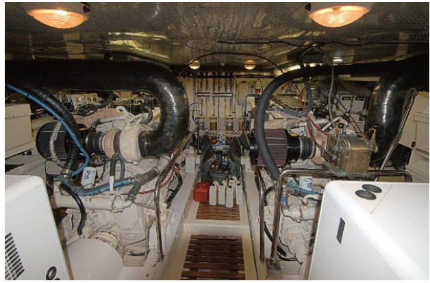
Engine Room Looking Forward
