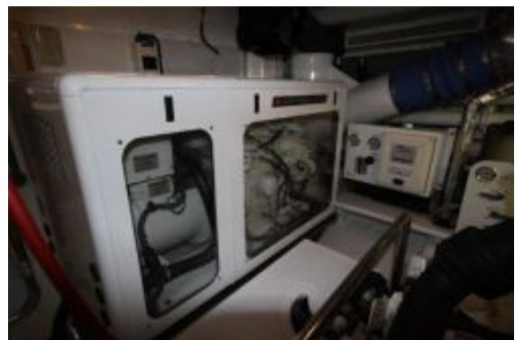
Northern Lights Genset
